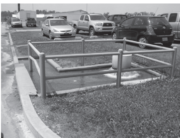
Discharge structure installed to discharge the sand boils near the LSU Vet School.
