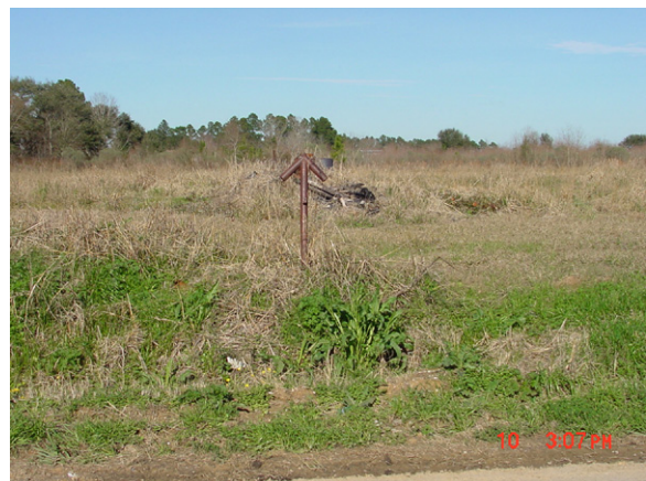
Figure 2.2.5 Unlabeled vent pipe
