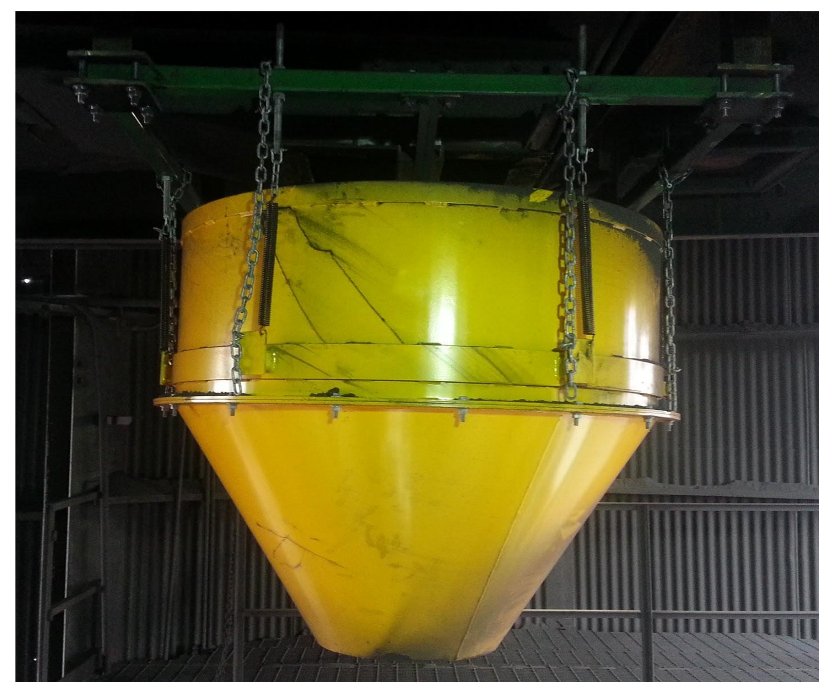
DSH Installed at Oxbow
