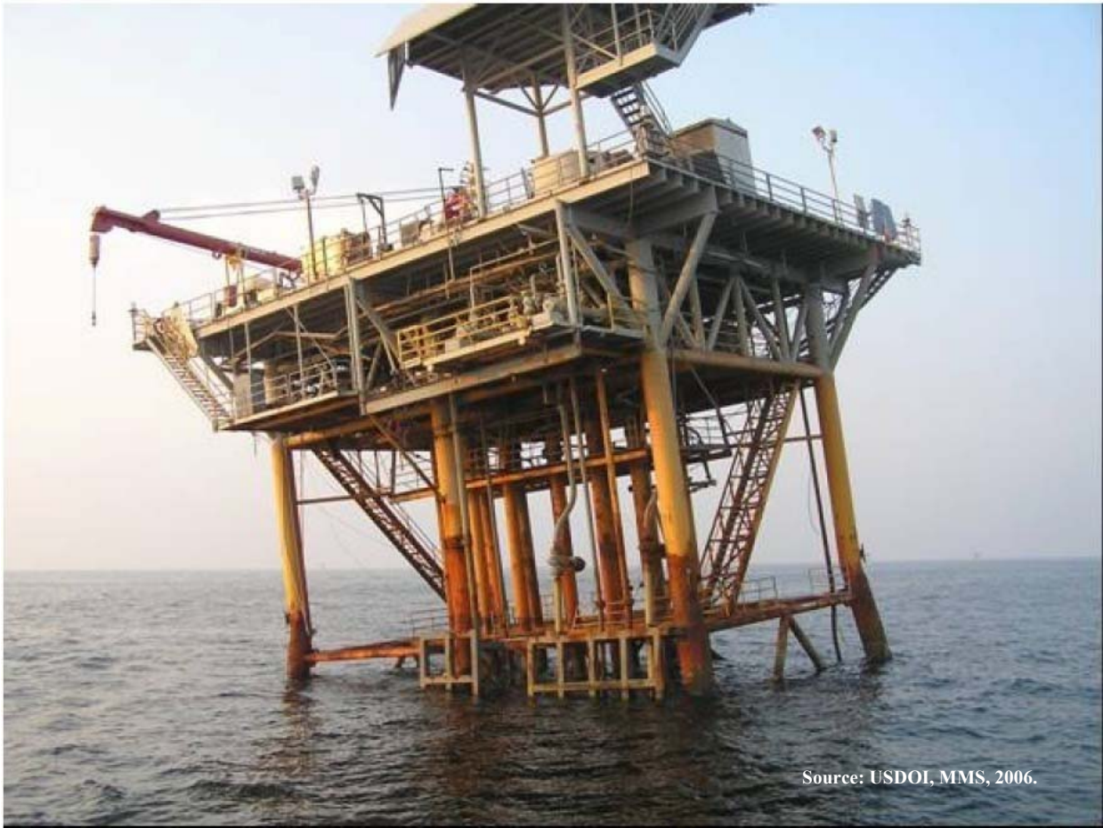
Figure A.3. Hurricane Destroyed Platform Suspected to Be Due to a Foundation Failure.
