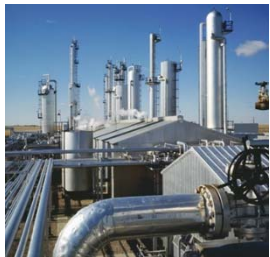
Natural Gas Processing
