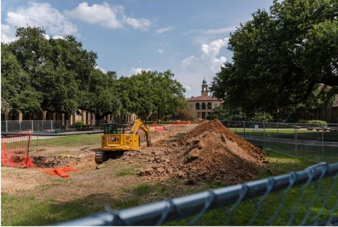
An excavator sits in a trench on Thursday, June 22, 2023, in the Quad on LSU's campus in Baton Rouge, La. Matthew Perschall
