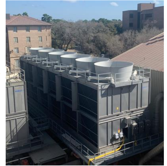
New Cooling Towers at the Powerhouse.
